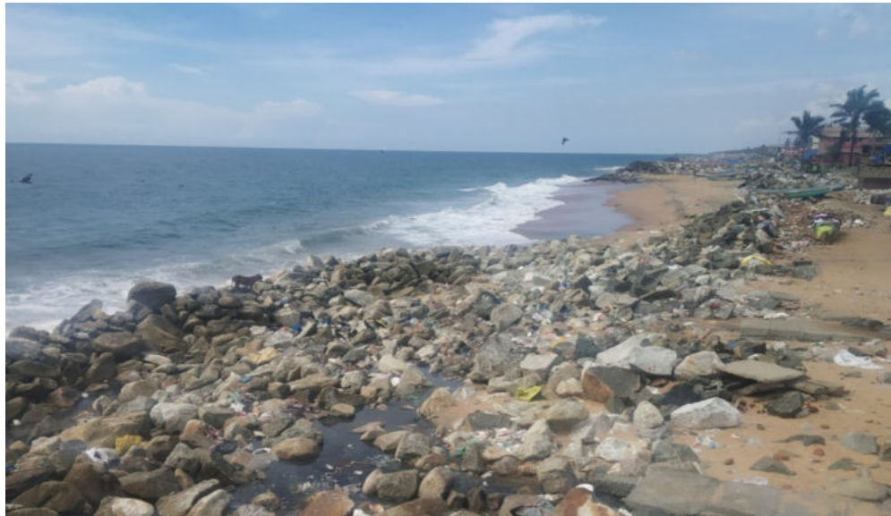
Damaged sea wall at Poonthura
