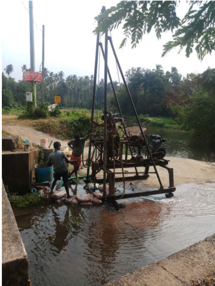
Soil investigation for the proposed RCB at Kainurchira, Nadathara GP, Thrissur Dt.
