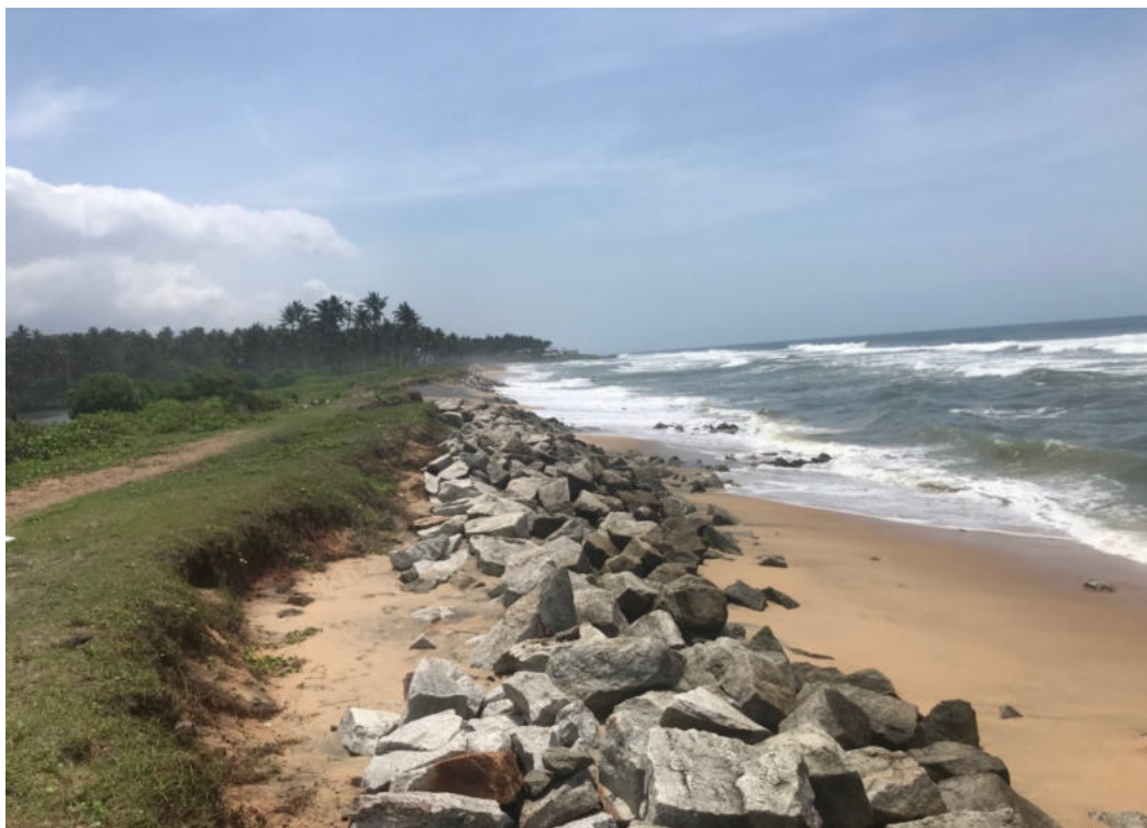
Damaged and collapsed sea wall at Edava
