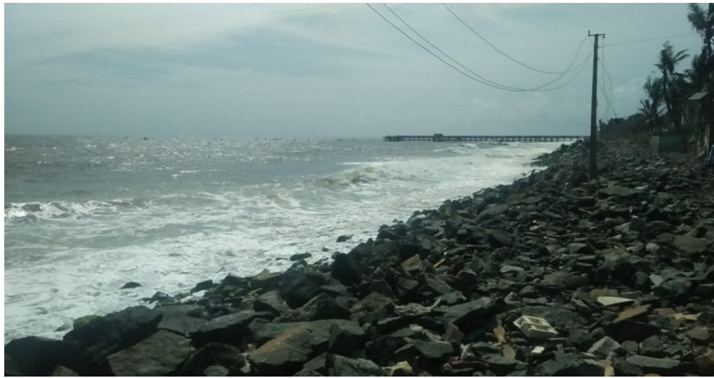
Damaged sea wall at Valiyathura
