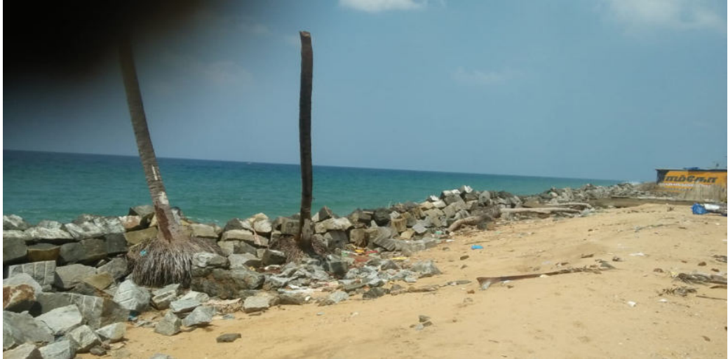
Damaged sea wall at Kollamkode
