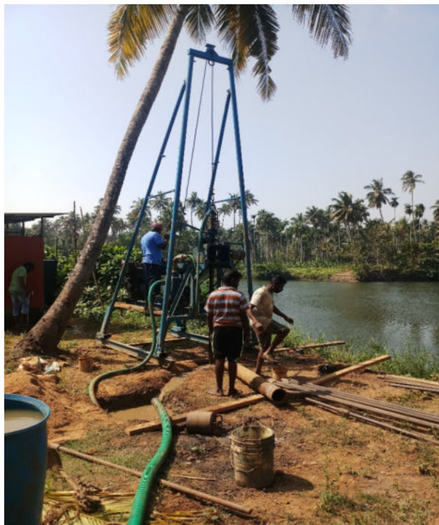
Soil investigation for theretaining wall & Approach Road of pro.regulator at Munayam, Thrissur
