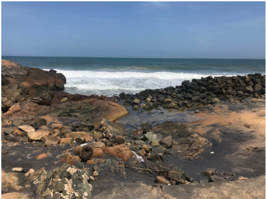
Damaged seawall at Samudra beach
