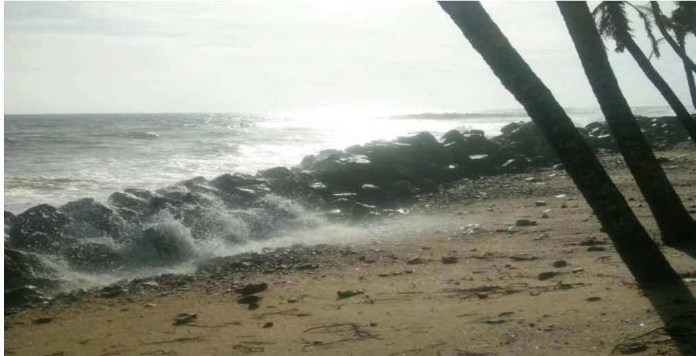
Damaged sea wall at Poothura
