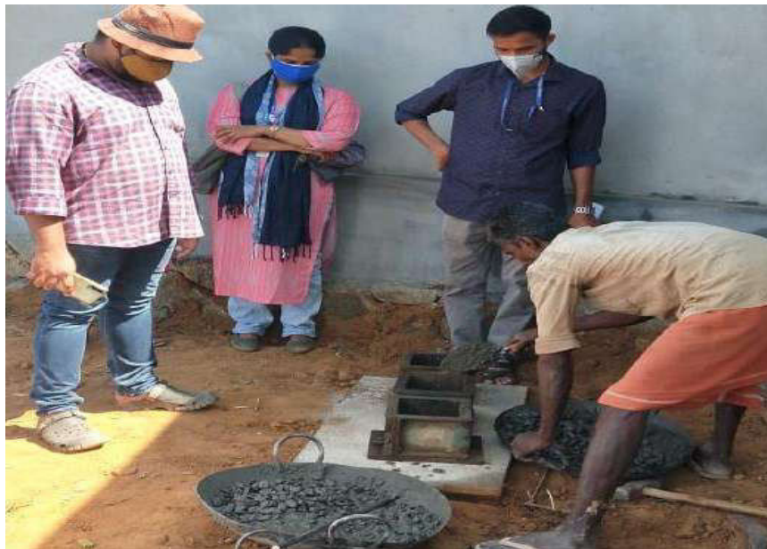
Sample collection from intermediate belt concrete of side protection wall under Irrigation section Changanasseri
