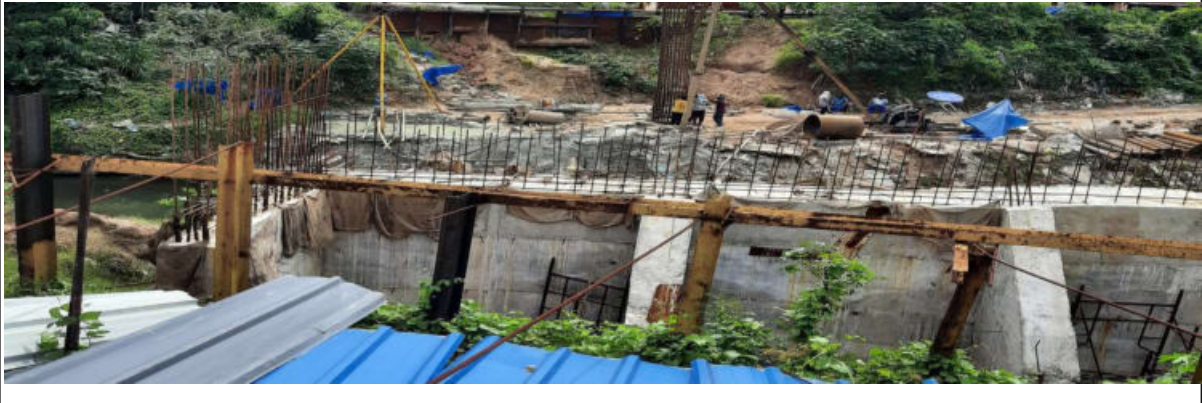
Pre- cast Pile concreting For Munroe Island Village Tourism Project.Irrigation Section Sasthamcotta.
