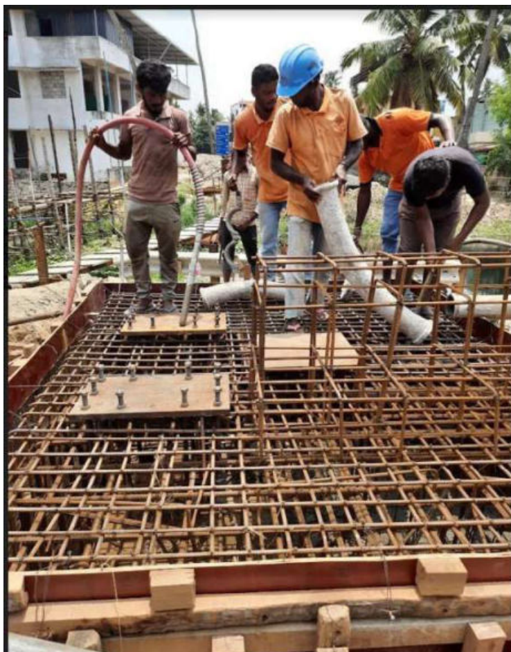
Pile cap for adjustable bridge at Karikkakom of Inland Navigation Section No. 3
